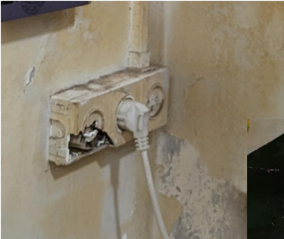
Broken plug socket
